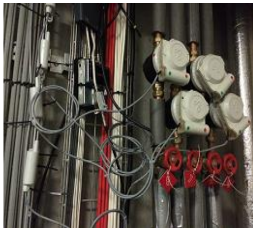
Photo 8: Example of congested nature of water supply pipes with sub meters
