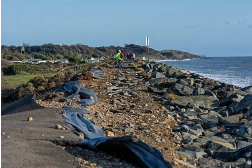
Figure 3.8: Dislodgement of pavement observed near the site after Storm Ophelia in 2017
