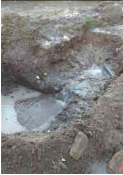
Photo 77: Southwest view of TP21, burst pipe.
