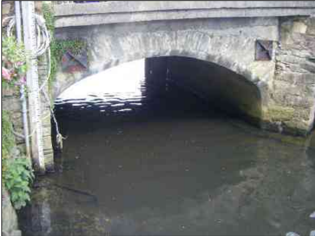
Figure 13 View of the southernmost span of Arklow Bridge (note the concrete encasement around the west abutment)
