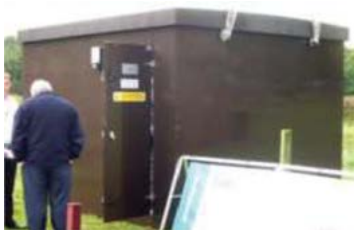
Figure 3 Typical orthophosphate dosing unit
