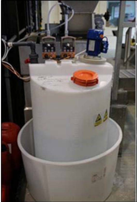
Hacketstown Water Treatment Plant Orthophosphate Treatment facility. Photo: Irish Water
