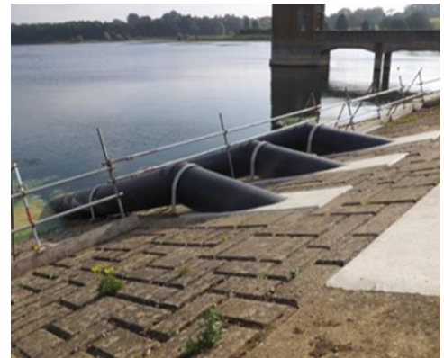
Figure 4 Example of a Siphon installation in a UK Water Supply Reservoir. (no railing proposed at Vartry)
